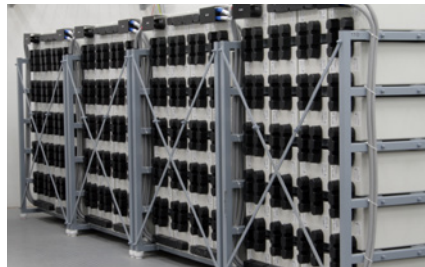
Energy Storage System
